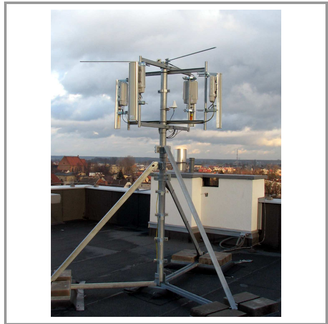
Fig. 1. One of INEA's WiMAX base station.
